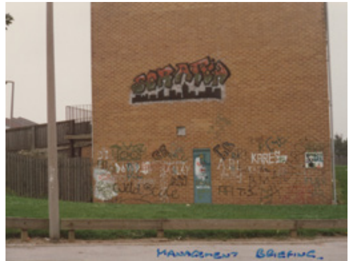
↑ Management briefing: vandalism at Trippett Court, Marmion Road estate (Courtesy Nottingham City Homes)
